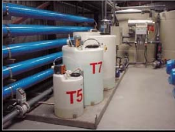
AMBR Post Treatment by Reverse Osmosis and Ultra-violet Disinfection
