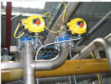
PROFIBUS and ASI integrated fieldbus control
