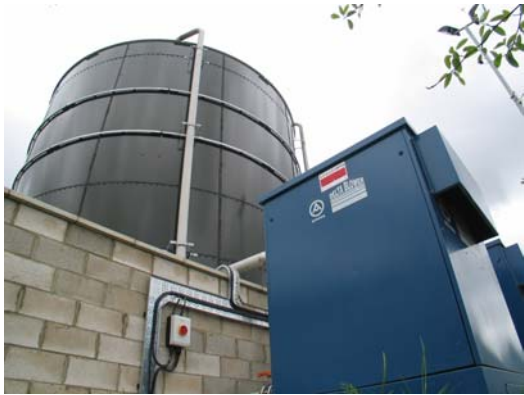
Figure 5 : AMBR Bioreactor, air blowers and JETOX aeration
