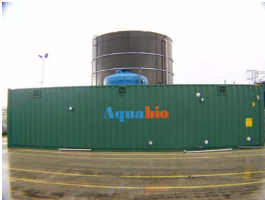
Figure 6 : Compact containerised plant for ease of expansion
