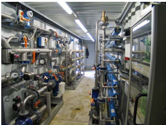
Figure 7 : The AMBR & RO membrane systems
